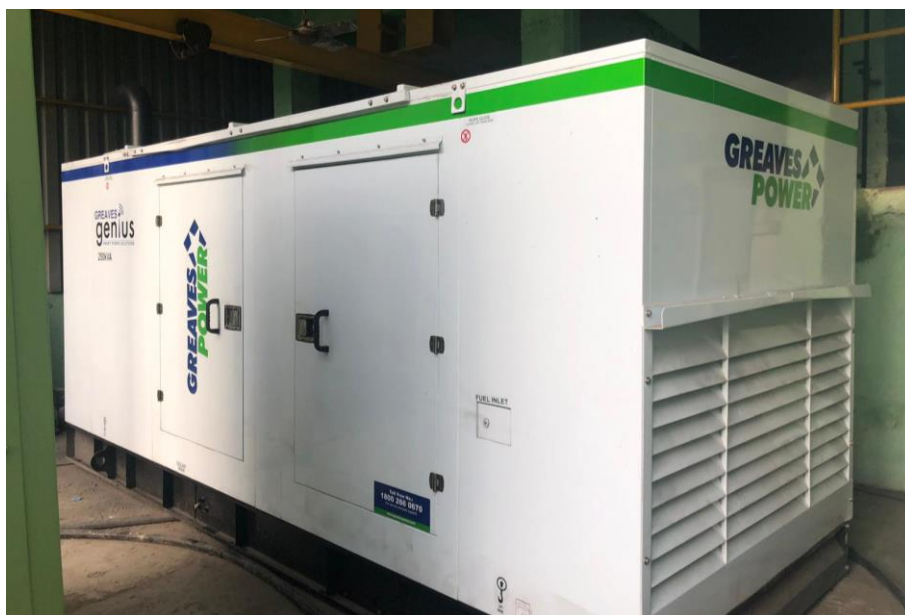
Figure 1 - Greaves Power GPW250 Diesel Generator.
